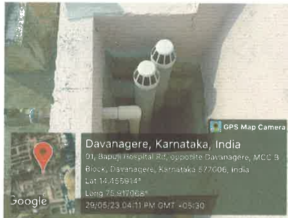
Photo 3 showing Concealed pipes from roof top to rainwater harvesting tank
